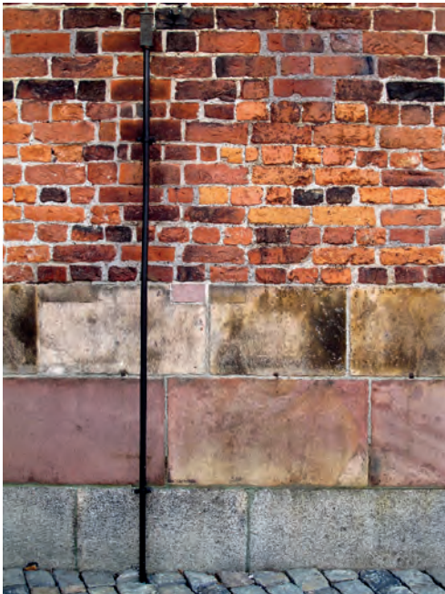
Fig. 14. Detail from the north wall of Riddarholmskyrkan, Stockholm shows how the brickwork starts above three courses of ash-lars. Photo: Morten Stige.
