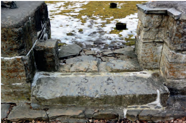
Fig. 9. The southern portal of the nave is the best preserved element of the Romanesque church. The portal is fitted with orthocer limestone. Photo: Morten Stige.
