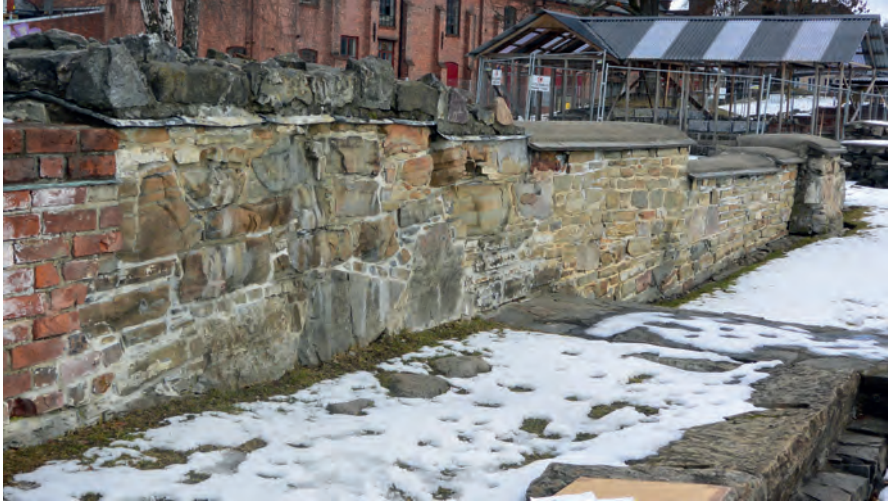
Fig. 8. Inner, northern wall of the nave displaying three periods of building. The Romanesque masonry to the right is cut and extended westwards by the Gothic elongation of the nave. Lastly, a later rebuilding in brick of the opening to the northern tower is seen to the left. Photo: Morten Stige.
