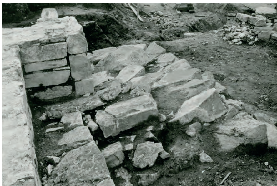
Fig. 25. The foundations under the Southwestern corner of the western tower show considerable settling stemming from the weight of the tower. Photo: Gerhard Fischer ( http://kulturminnebilder.ra.no ).
